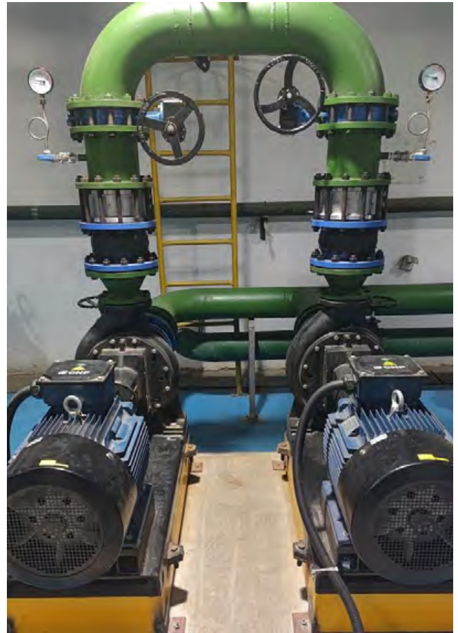
Photo: Hangzhou, China Renovation of independent water supply by air compressor at the Yuhang plant.
